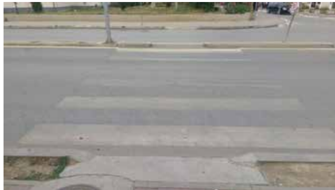
Figure 3. Typical example of pedestrian crossing that does not meet the standards
